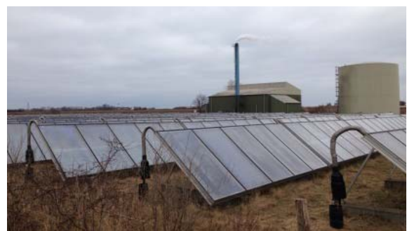
Figure 2: Nordy-Mårup district heating plant
